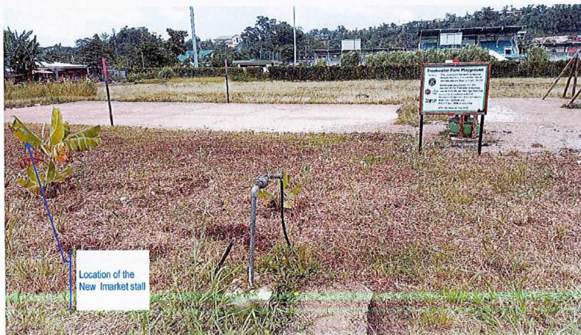
Plate 15: Existing volley ball court to be rotated (partially reconstructed) in order to be fully outside the construction area and location of the new small market stall (food stall)
